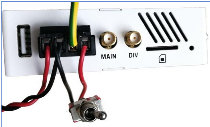
Screenshot 3 Installed RAR with switch at digital input 1.
